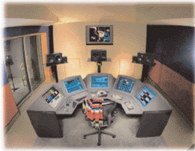
DSP's Postation (circa 1998) installed in Margarita Mix studios.
